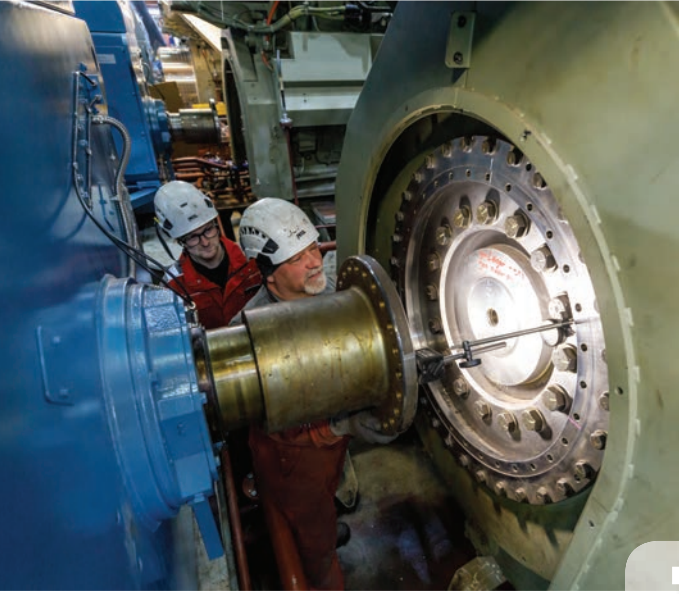
LINE IT UP: Alignment of one of the new main engines (right) with generator (left).
