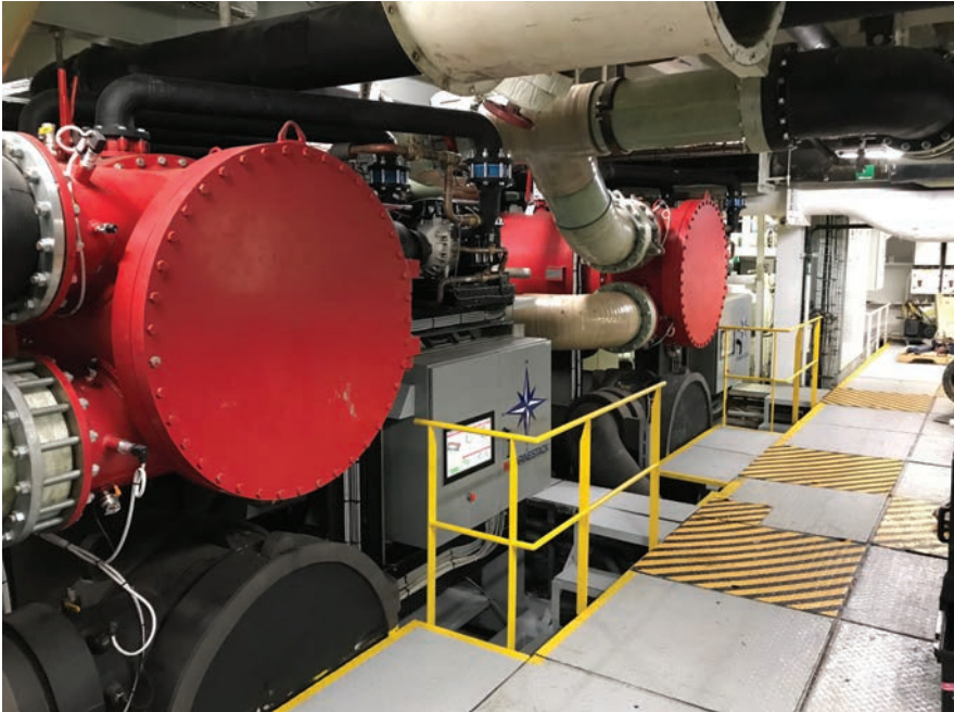
The chiller solution provided to RCCL by Multistack.
