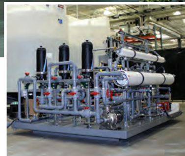
Water Recycling Technologies
