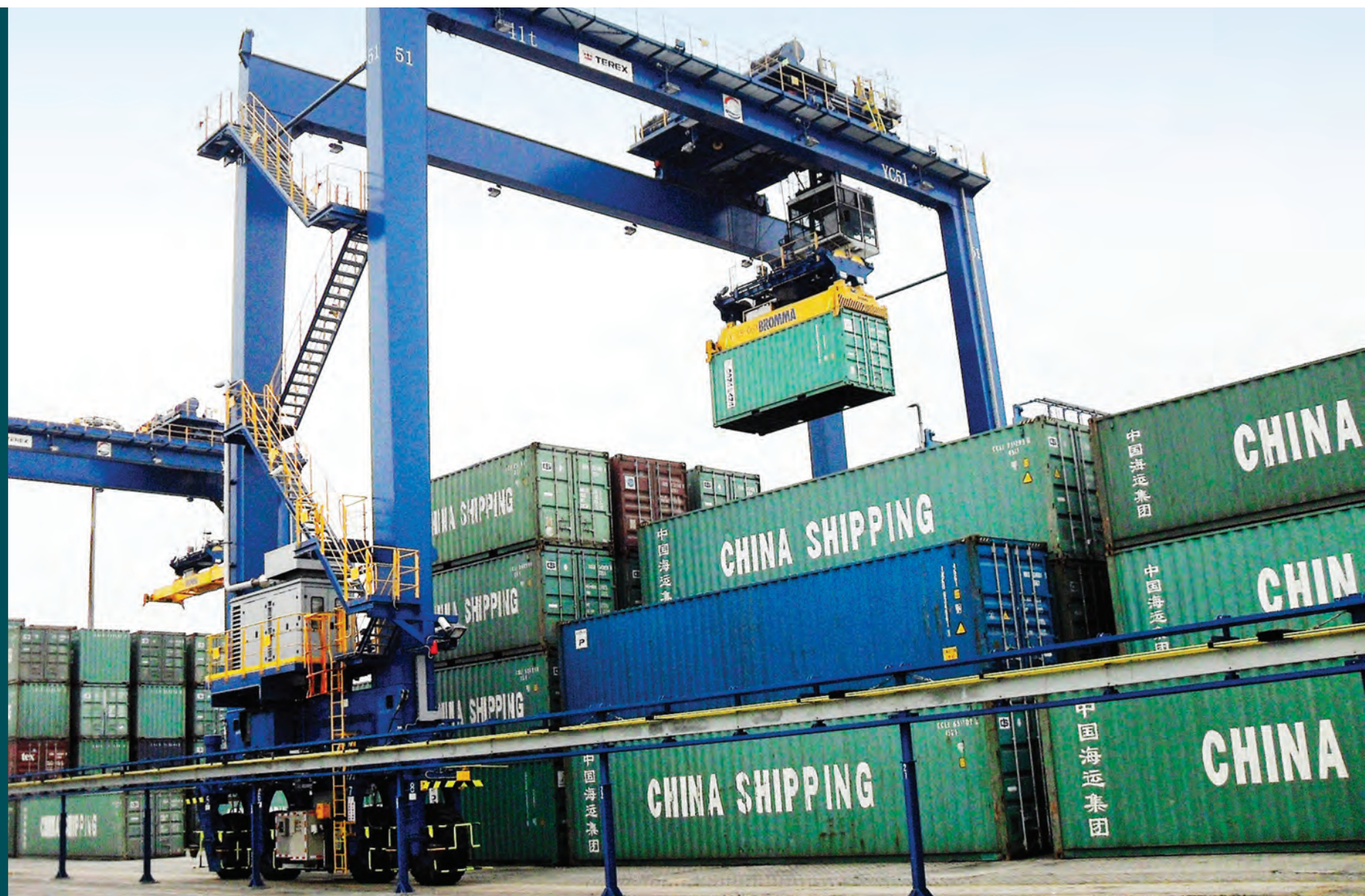
The PBES/CCCC Shanghai RTG hybrid battery crane in Shanghai, reducing emissions from port operations.
