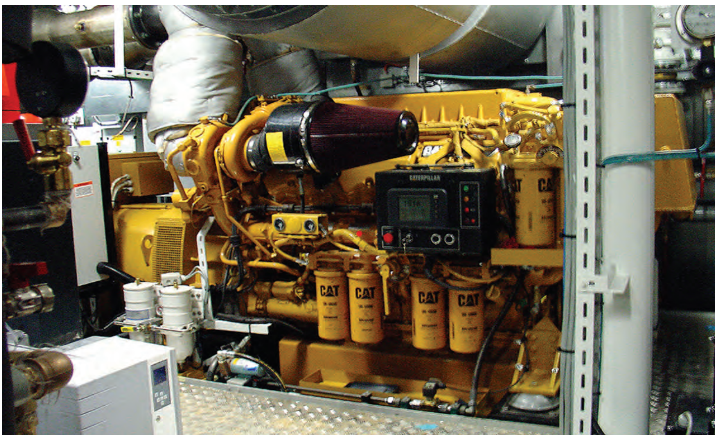
Generator in the engine room.
