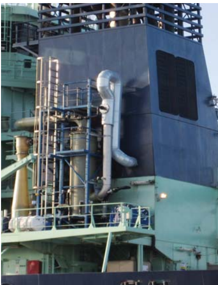
Figure 1: Exhaust gas scrubber onboard the MT "Suula".
