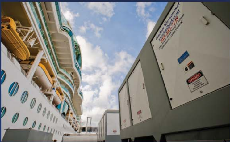
CR922 Medium Voltage Load Bank
