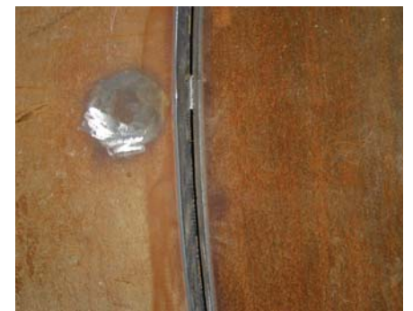
Pipe cutting and beveling tolerances on the project had to be held to within 1/16 inch per foot of diameter with a maximum allowable deviation of 1/4 inch.
