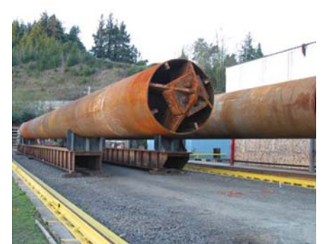
The pipes shown on this jig stand are ready for extension pipe fit-up.
