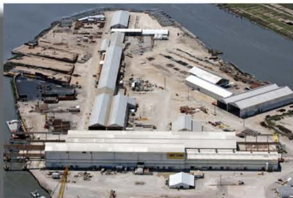
Above photos depict the ongoing construction of two 300' x 100' power barges at Signal's Orange facility.
