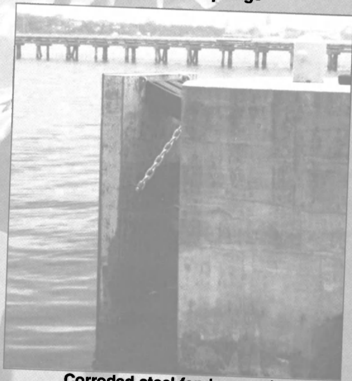
Corroded steel fender panel
