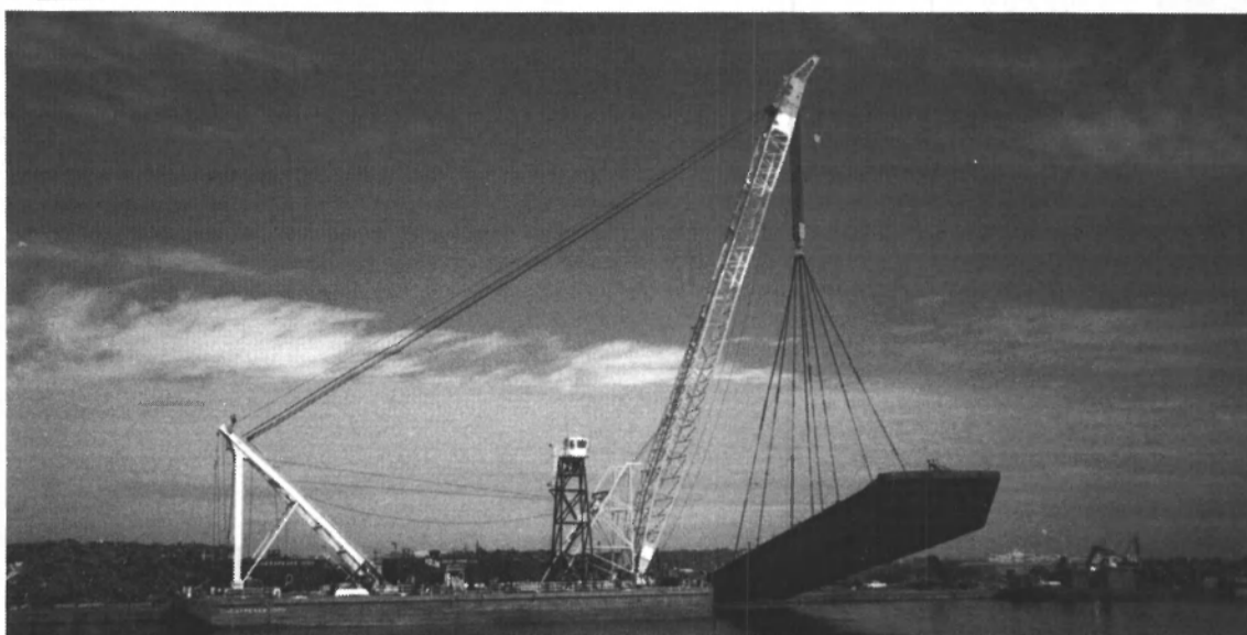
Derrick Barge CHESAPEAKE 1000
