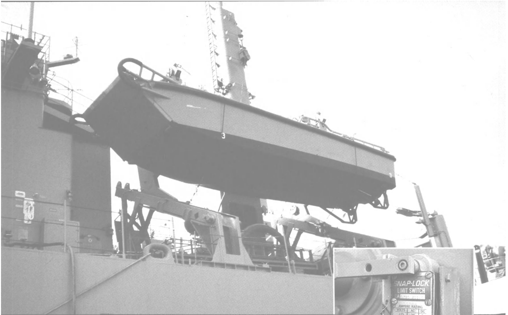
Mechanical limit switches are still preferable to electronic proximity switches in most Navy applications. Here, a Namco Snap-Lock® switch controls a davit gearbox. Rugged Snap-Lock switches have reliably stood up to harsh environments like this for years.
