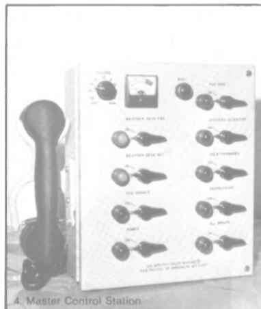
4. Master Control Station
