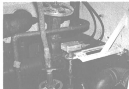
Typical RMVA installation, valve end after one year of operation
