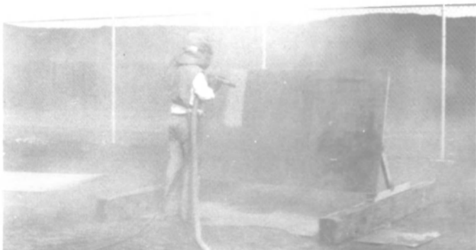
Dust (shown here from silica sand) means lower cutting efficiency and visibility and increased health hazards and clean-up costs.
