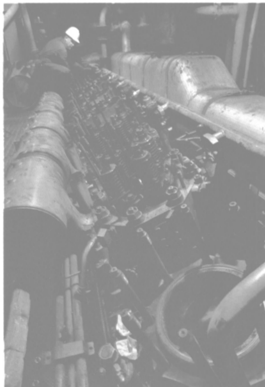
The port engine during overhaul and inspection.
