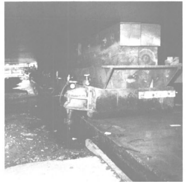
Connections and hoses under barge lead to Aero-Caster water bearings placed directly on concrete runways. When water bearings are inflated, they create a film of water to float barge along runways during transfer. The 96 Aero-Casters used to move the barge were made by Aero-Go, Inc., Seattle, Wash.
