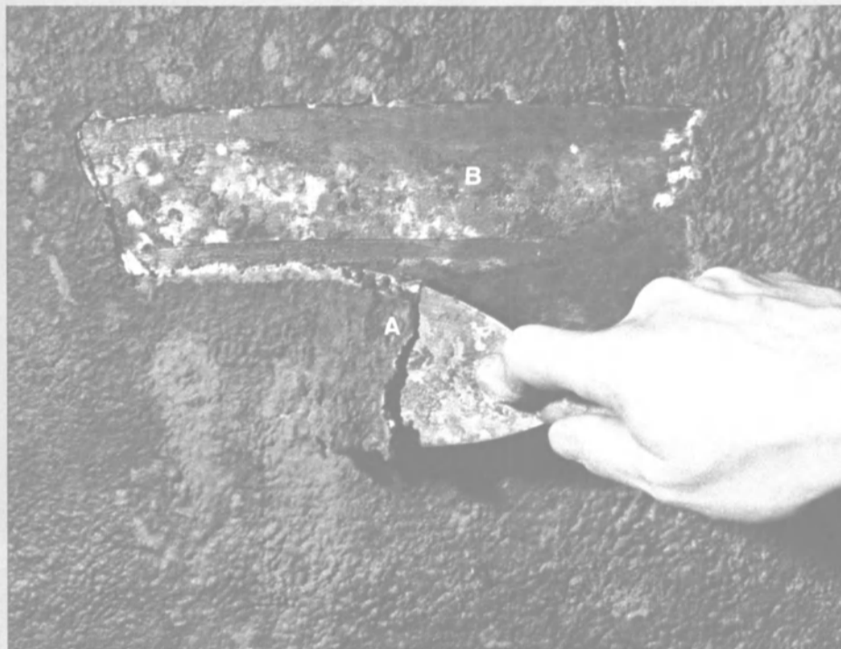
Photo from ABSTECH report shows no rust damage after 9½ years. When Fluid Film (A) was scraped away from ballast tanks, no oxidation was found on base metal (B).
