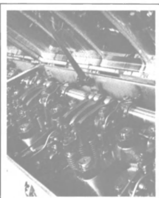
Valve deck illustrates cleanliness typical of both engines.
