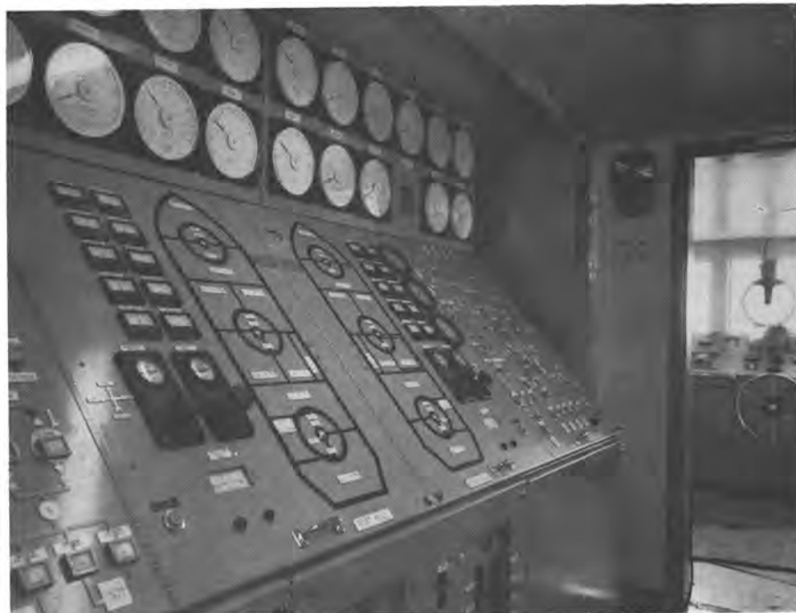
Central control panel of Pacesetter I, located adjacent to pilothouse, employs sophisticated instrumentation to monitor operation of the drilling unit. The console shown controls all pumping of hull tanks, with continuous registering of the amount of fluid in each tank visible on the circular gauges seen at the top of the picture.
