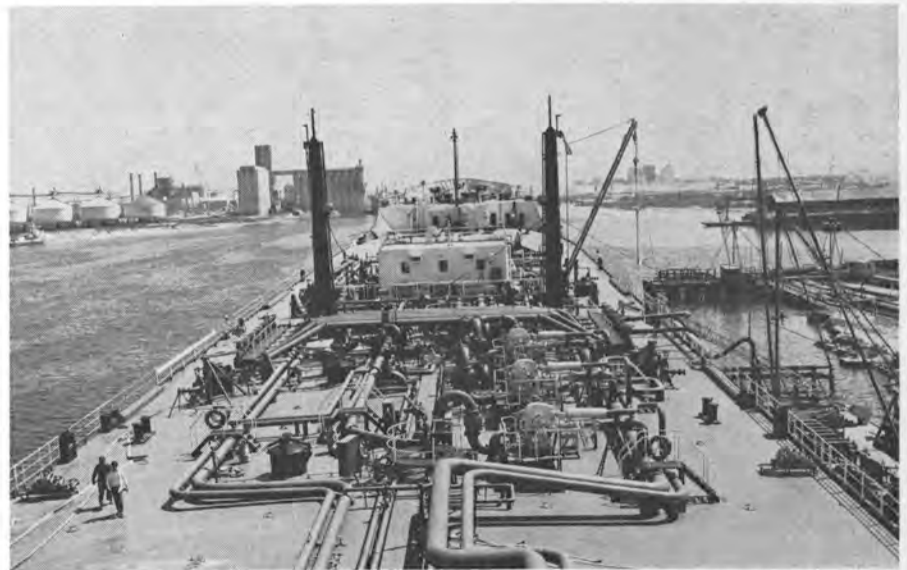
View of the main deck clearly shows three of the deep-well pumps on the starboard side.
