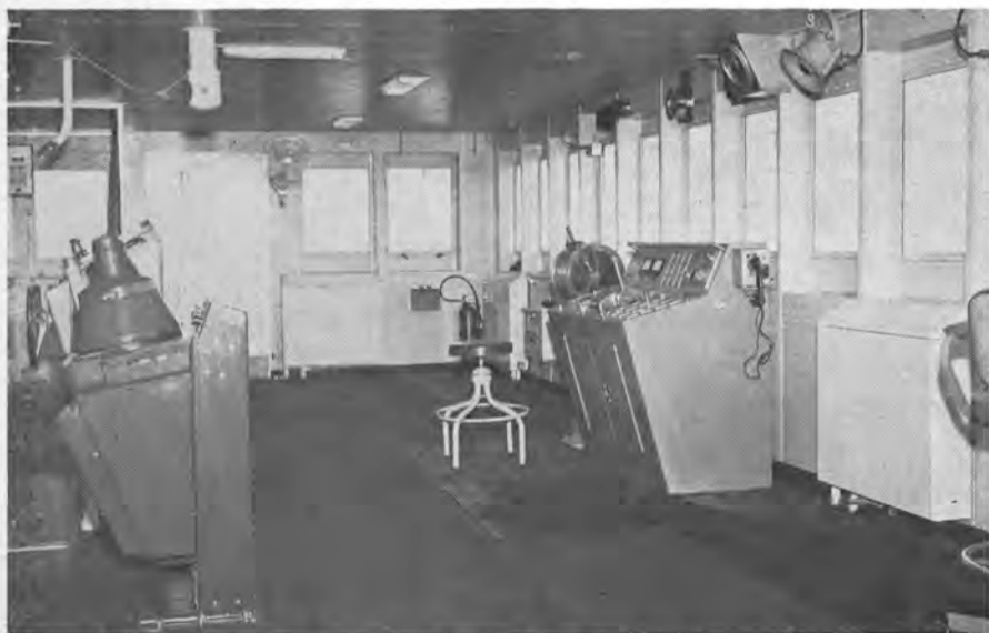
The Falcon Lady's pilot house has engine controls located along the forward bulkhead.
