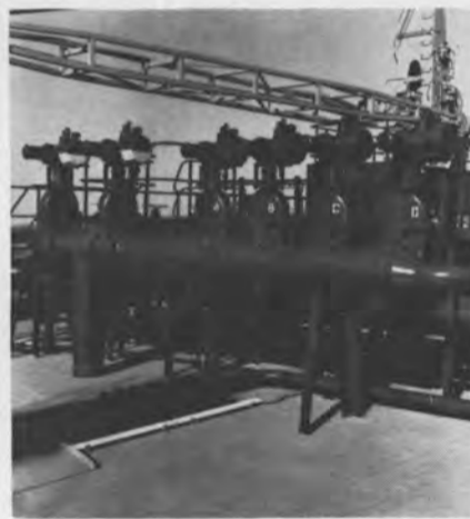
Remotely-controlled manifold valves on deck.
