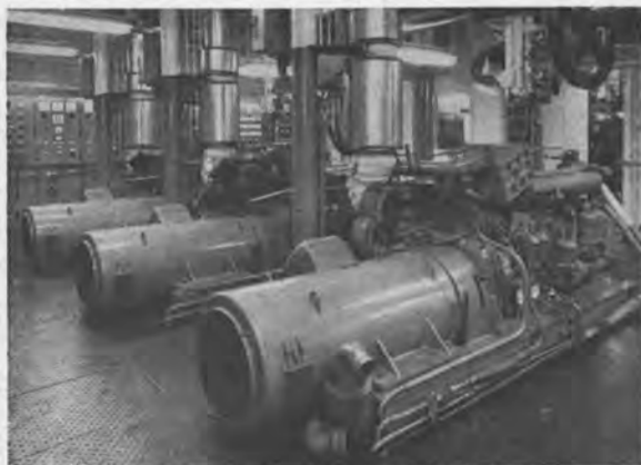
Electrical power is supplied by three diesel-generator sets.
