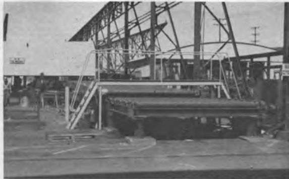
Figure 4—The Tee welder receives cut plates by transfer car from flame planer and welds them into beams.
