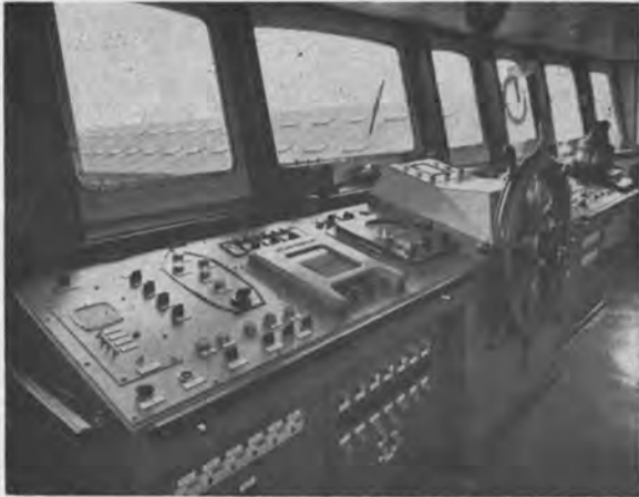
Pilothouse console combines all ship operating functions.
