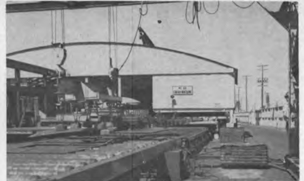
Figure 5—The CM 60 machine performs profile cutting operations. Magnet lift removes scrap material.
