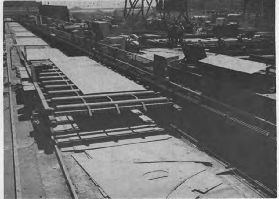
Figure 2—The Collocator receives material from either of two transfer cars and distributes it at assigned locations along 1,000-foot track for subassembly and forming.
