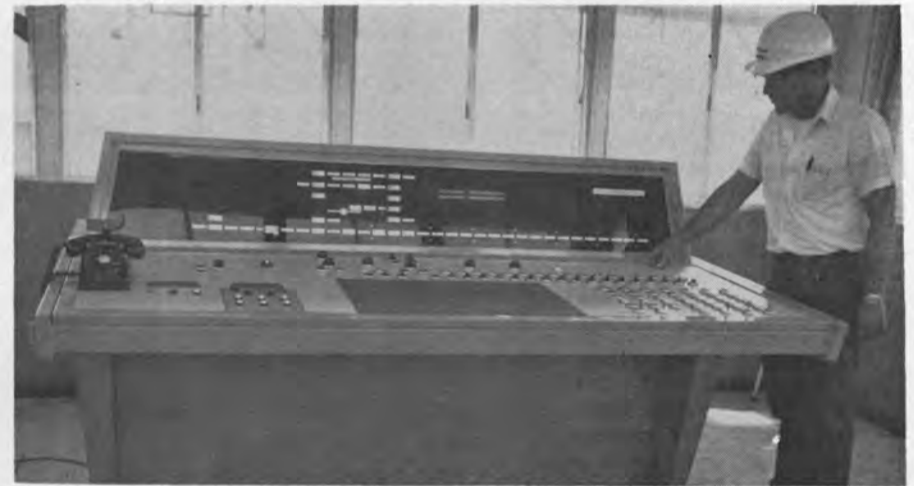
Figure 7—Central control console can handle all material transfers in programmed sequence or transfer control to local stations. Located in an elevated tower, it permits the operator to have full visual view of operations.
