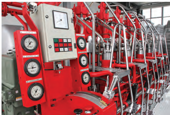
The New PrimeServ Academy in Copenhagen is the only engine school in Europe equipped with a full size 2-stroke engine of type 6S35MC, which has been built at Alpha Diesel in Frederikshavn
