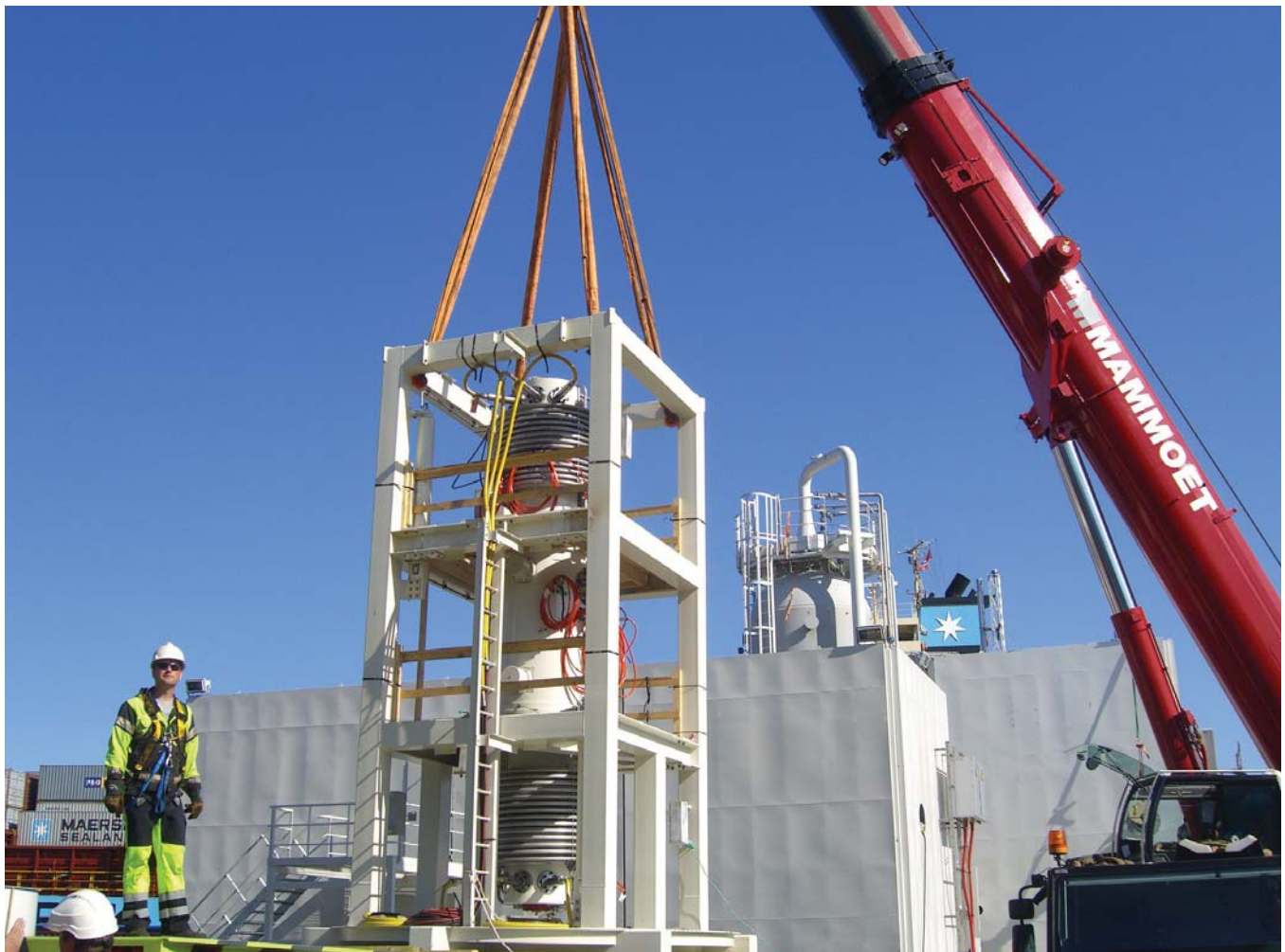
Framo Engineering's Wet Gas Compressor unit hanging from a crane prior to installation in the test loop tank.
