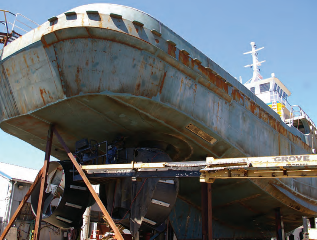
The latest Titan class tug under construction at Western Towboat is scheduled to launch in late October. The bilge keels visible toward the front of the hull help offset the "rolly" effect of the hull shape necessitated by the Z-Drives.
