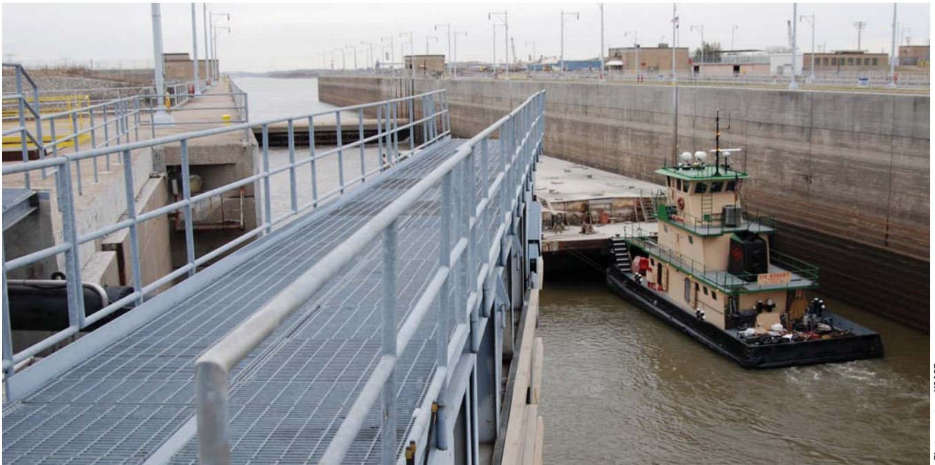
One of the two miter gates of the auxiliary chamber close behind the M/V Sir Robert at Locks 27 in Granite City, Ill.
