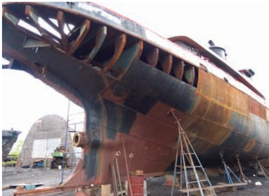
Hull plates and frames and bulkheads all had portions that were "worrisome," requiring the calming effects of work such as this a year ago. (Photo: Don Sutherland.)
